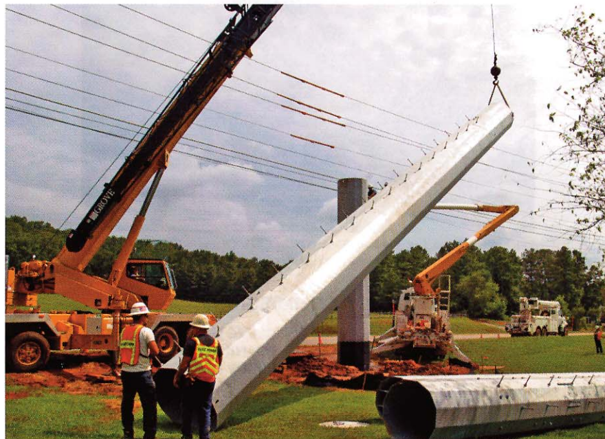
Hardhats, cranes and bucket trucks are a common sight as the state's utilities build out the power grid to keep electric reliable. Georgia Transmission's crews installed this transmission line a few years ago to prevent overloading of the transmission system in Forsyth and Cherokee Counties.
