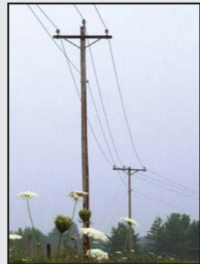
25 kV or 12 kV
