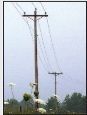
25 kV or 12 kV
